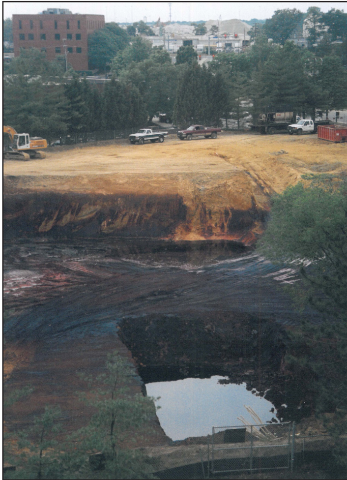
Chafferty's site after excavation and completion of groundwater remediation with backfill of #57 stone layer.
